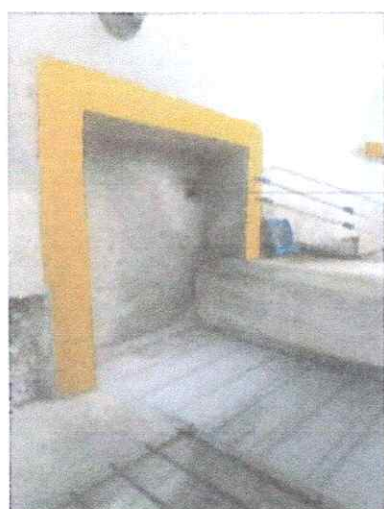
EXIT DOOR ENCLOSURE 1 FLOOR DRAIN WITH 4" PVC DRAIN PIPE TO EXISTING DRAINAGE
